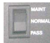
Switch in Normal position
